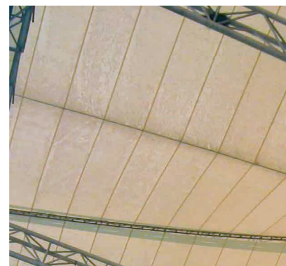
Image 2: Lacquer adhesion problems in translucency. Where lacquer is not performing the coating is directly exposed to soiling and UV attack.
